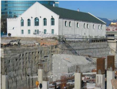
"The forty foot drop-off at the rear of the Drill Hall....2004"
